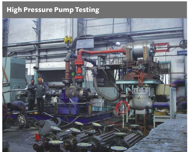
High Pressure Boiler Feed Pump Testing facility at Poona, India controlled by an MIL MATRIX Series Valve. Here the valve is used to kill high pressures generated by the Boiler Feed Pumps, which can be as high as 420 Kg/cm 2 .
