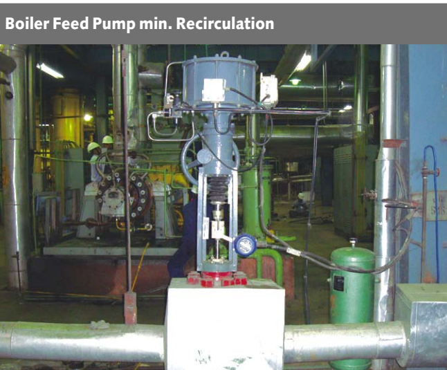
Thermal Power Plant in Orissa, India with MIL MATRIX Series valve controlling the BFP Min. Recirculation Flow. These valves have 25 Pressure/ Velocity Reduction Stages and a strainer in-built to the seat, which protects Trim from foreign material.
